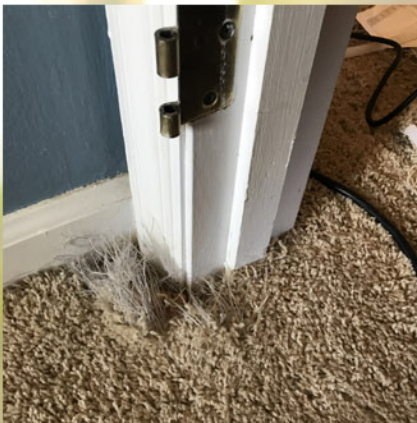
PET DAMAGE TO CARPET BY DOOR
