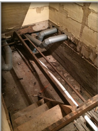
EXISTING SPACE ROTTING FLOOR AND STRUCTURE
